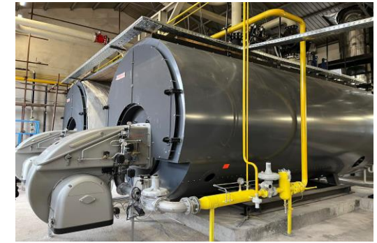
Gasna kotlovnica (2 x 10 MW)
